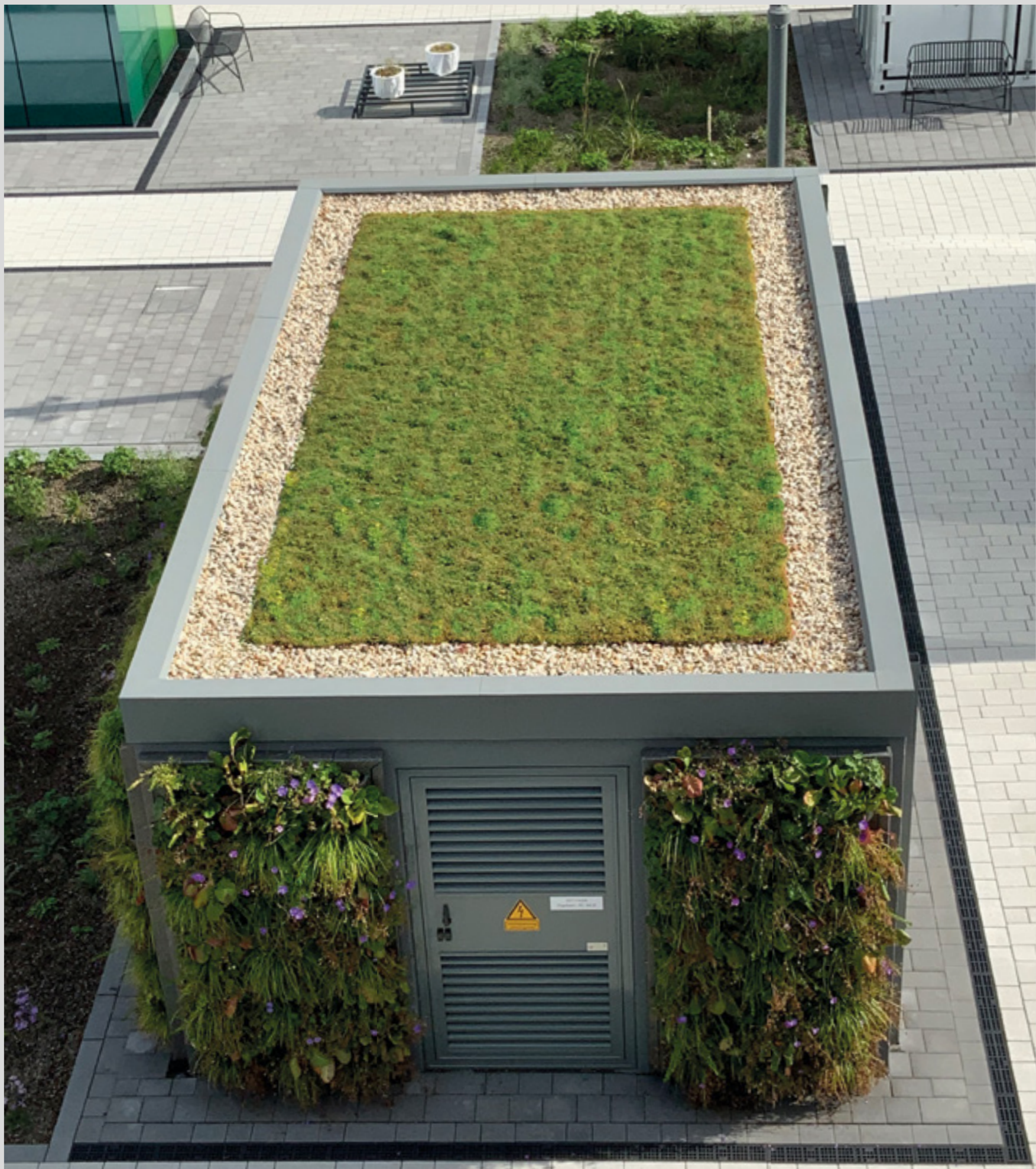
Trafostation; Phoenix All Elektrik Society Park Blomberg
