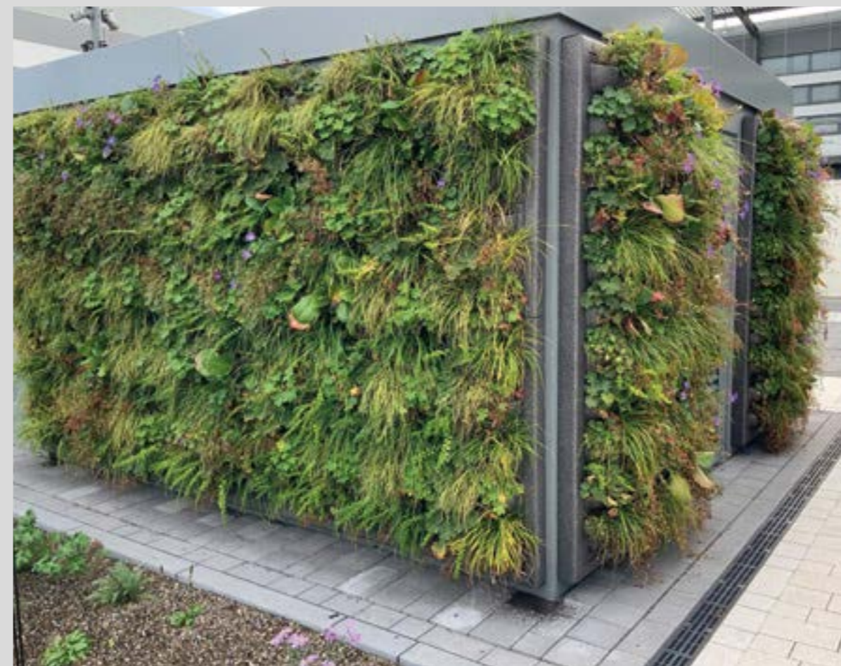
Trafostation; Phoenix All Elektrik Society Park Blomberg
